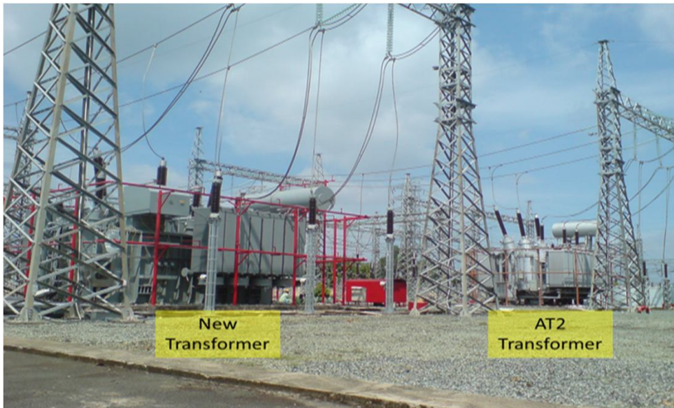
Installed and commissioned secondary back-up transformer at 220KV Cat Lai power station, further enhance reliability and flexibility of power supply
